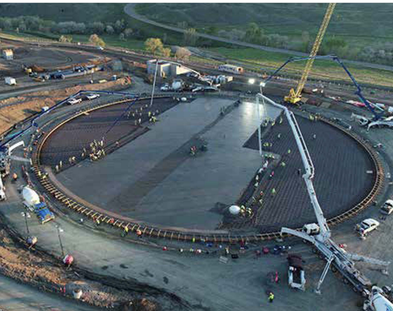
Northwater Treatment Plant
